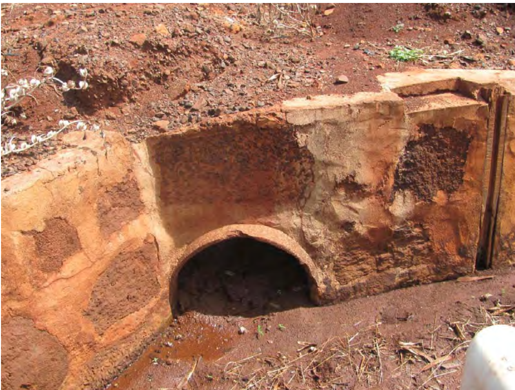
Figure 138. Site 7170 Section 13 where concrete pipe enters from Section 12 and an old sluice is present, view to the east.
