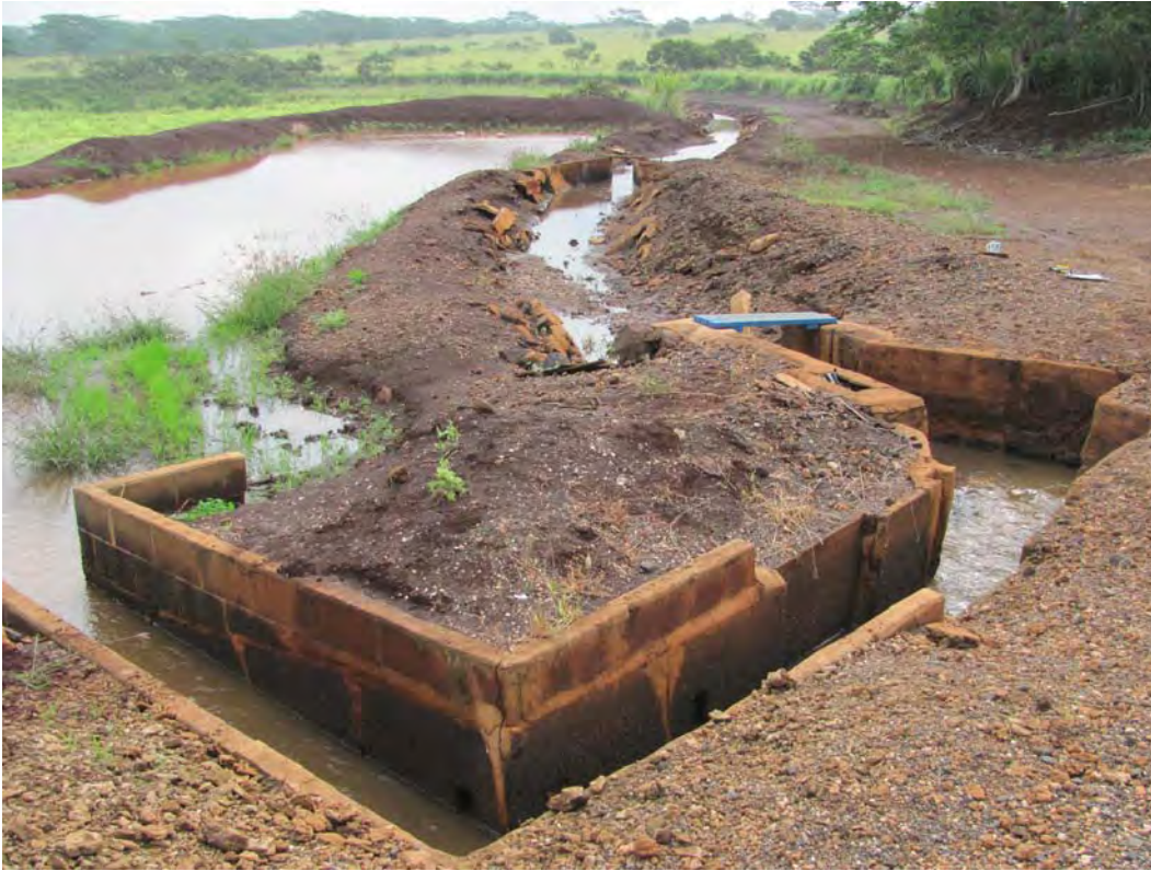
Figure 65. Site 7159 Section 7 sluice gate complex north of Kawailoa Road, view to the north.
