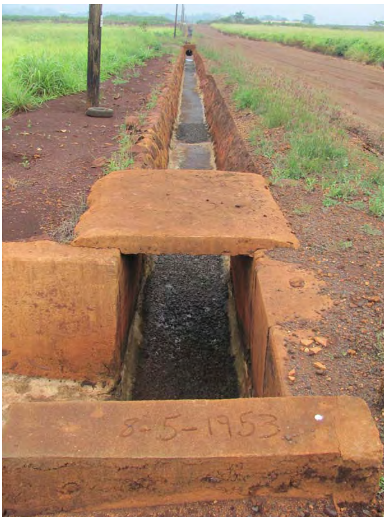
Figure 67. Site 7159 Section 9 sluice gate complex at start of section, view to the southwest.
