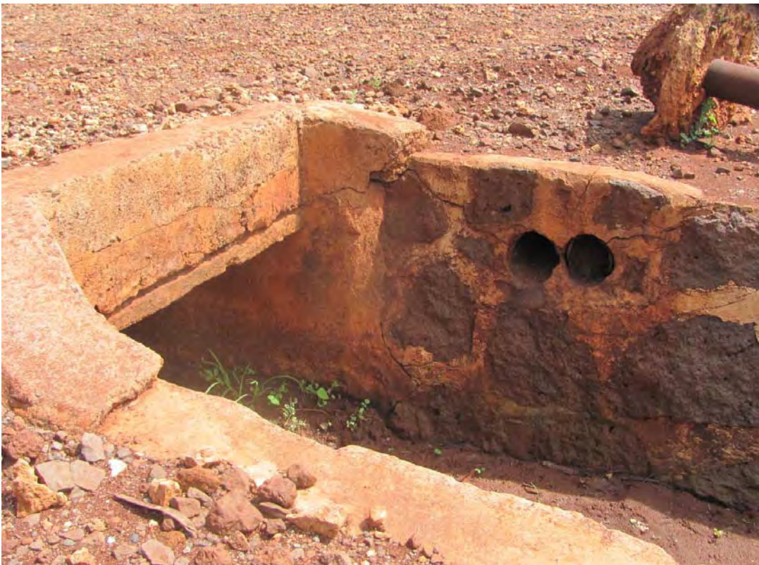
Figure 141. Site 7170 Section 14 metal pipes near the northeast end, view to the northeast.
