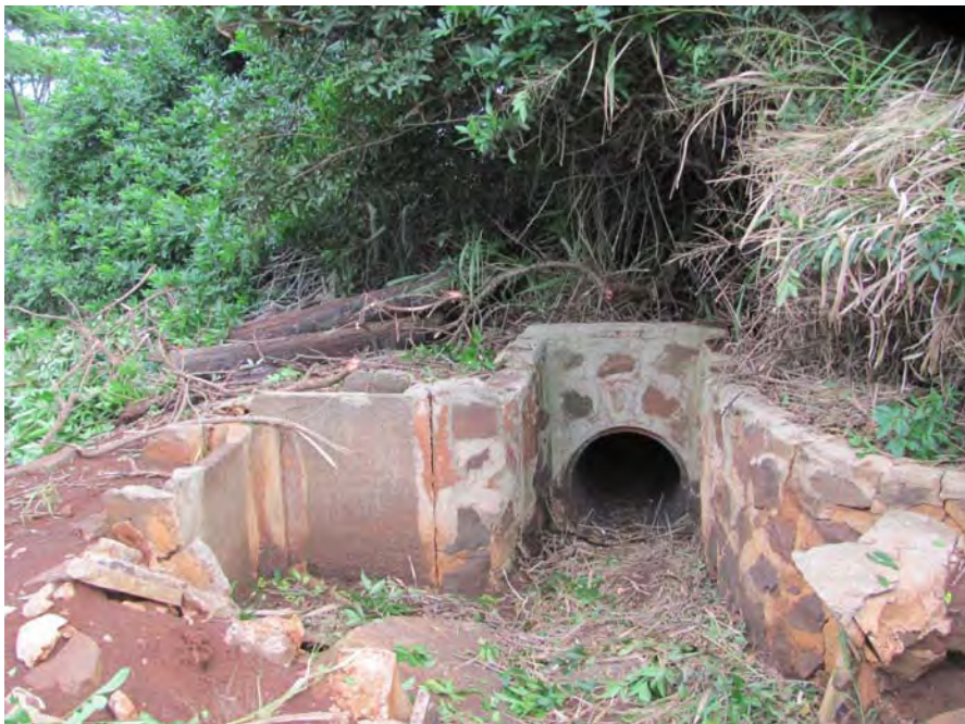
Figure 104. Site 7169 Section 1 sluice gate complex at north end, view to the northeast.
