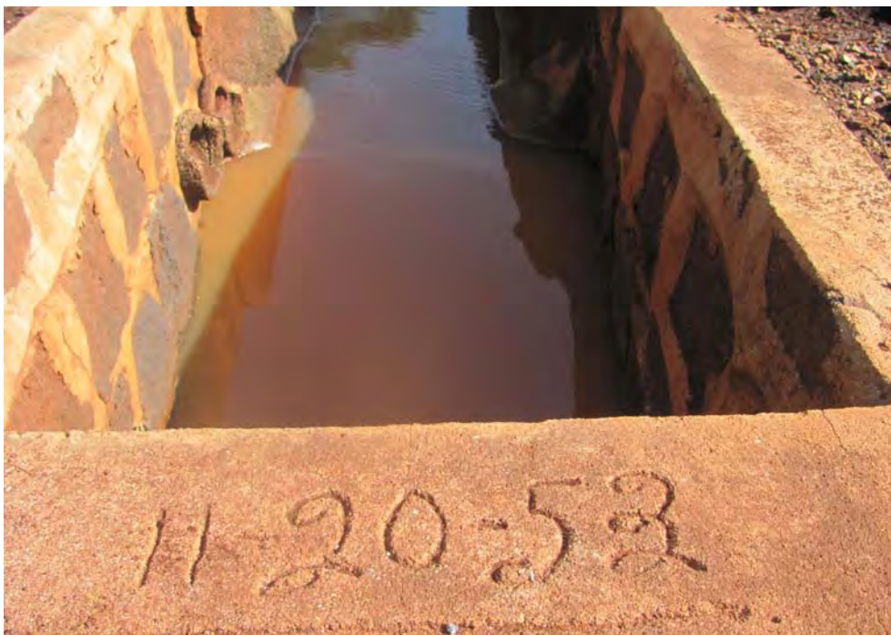
Figure 115. Site 7170 Section 1 date inscribed in concrete at south end, view to the northeast.
