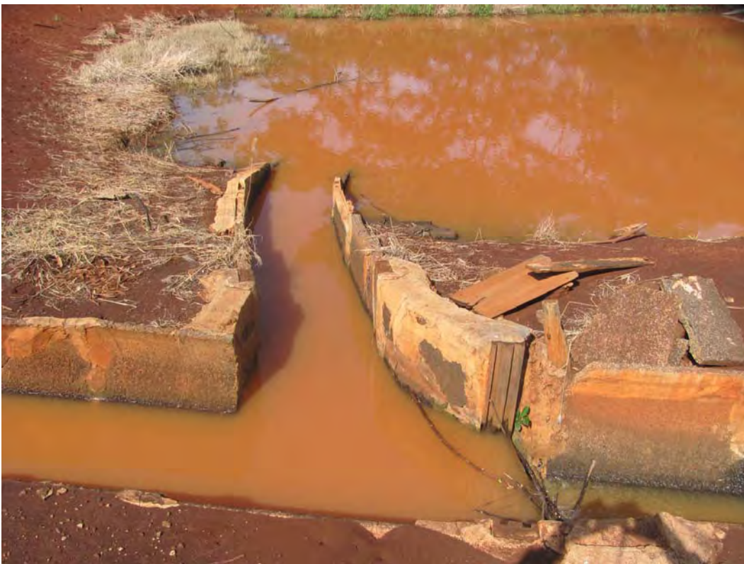
Figure 119. Site 7170 Section 2 sluice and channel leading to the water retention pond, view to the west.
