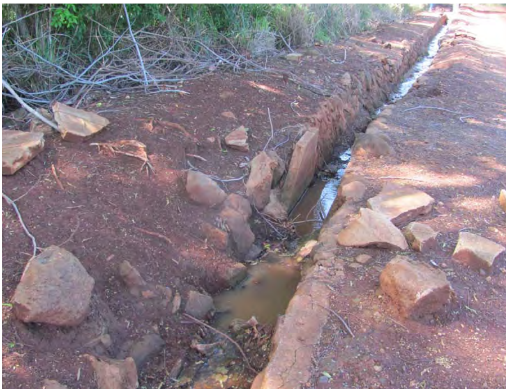
Figure 128. Site 7170 Section 8 concrete retainer in south wall of ditch, view to the southwest.
