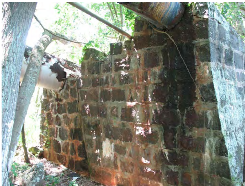
Figure 92. Site 7164 piers supporting the upper section of the pipes, view to the northeast.
