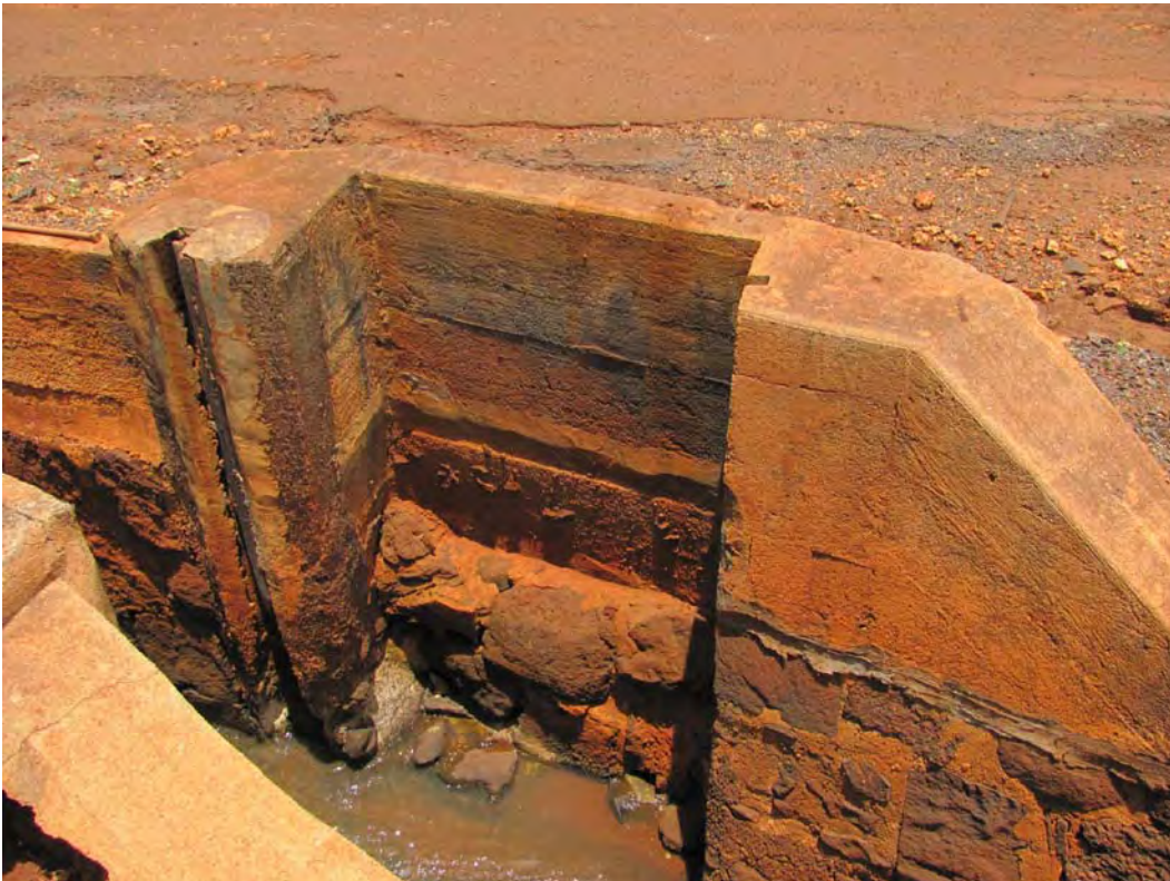
Figure 61. Site 7159 Section 7 sluice gate complex at start of section, view to the north.
