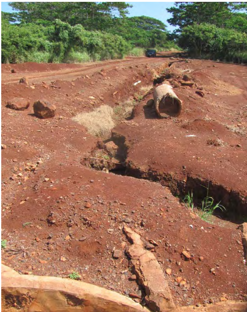
Figure 136. Site 7170 Section 12 eroded makai end, view to the east.
