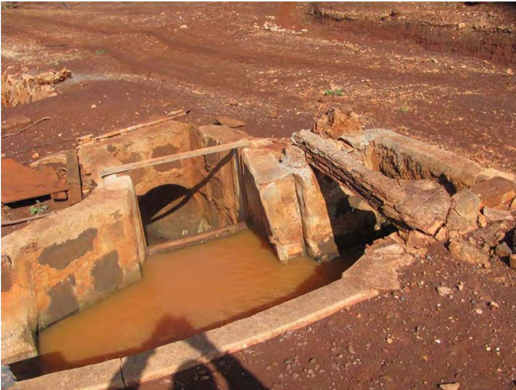
Figure 116. Site 7170 Section 2 sluice gate complex at Mid-Line Road, view to the northwest.
